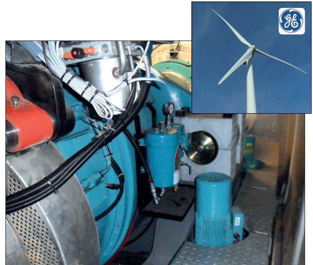
CJC™ Fine Filter HDU 15/25 PV2 installed at North American Wind Research and Training Center
