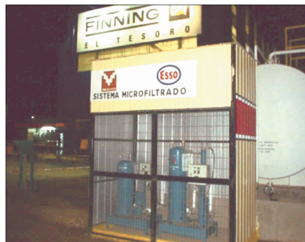
CJC Filters installed in Minera El Tesoro.
