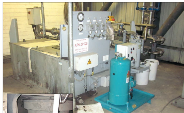
Coal Mill, Ireland, Gearbox, MAAG Gear with installation of CJC™ Fine Filter HDU 27/54 PV
