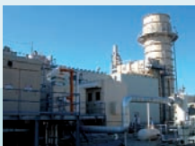
Major Electric Power Plant, USA
